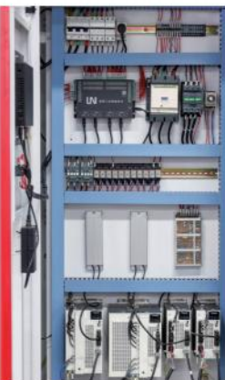
Electric cabinet with Schneider parts
